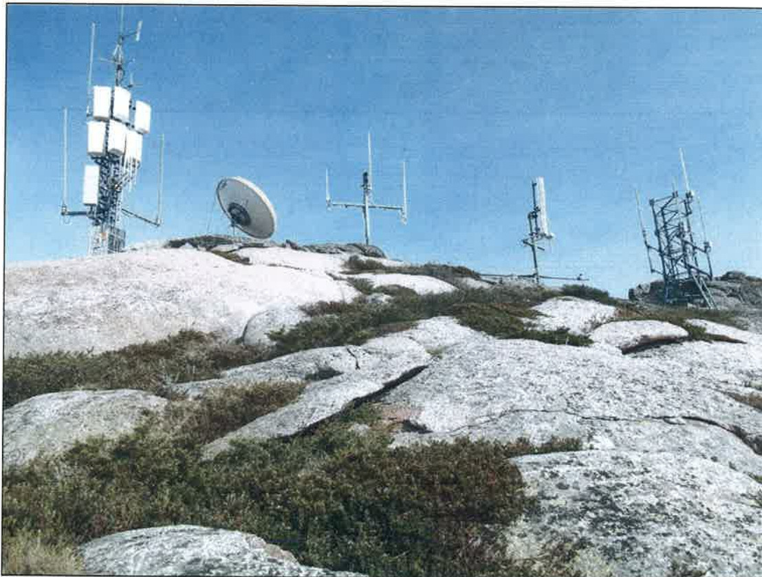
Photo 3: Existing telecommunications facility at Eagles Nest.
